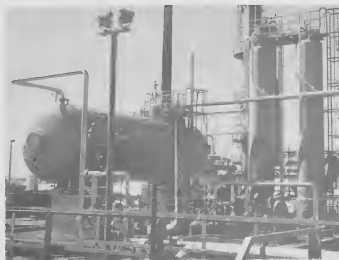
THE LEAR Mercox Unit at left went on stream recently. This compact and efficient unit will replace the Cracked Sweetening Plant, at the right.
